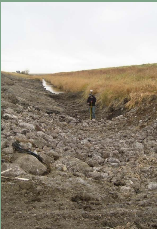
Judicial Ditch 75 grade stabilization in 2020
