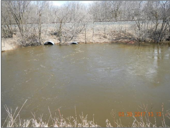
Figure 2-4. Railroad culverts inundated (Downstream Side)
