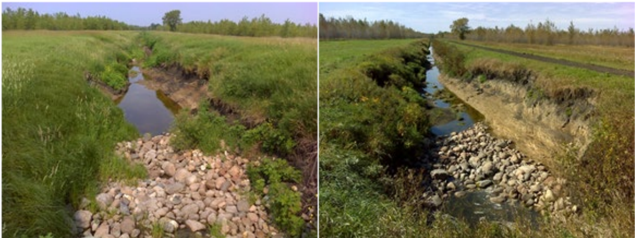
Figure 56. Images of a rock check dam at the 480 th Avenue NW crossing along AUID 519 on July 1, 2015 (left) and September 21, 2016 (right).
